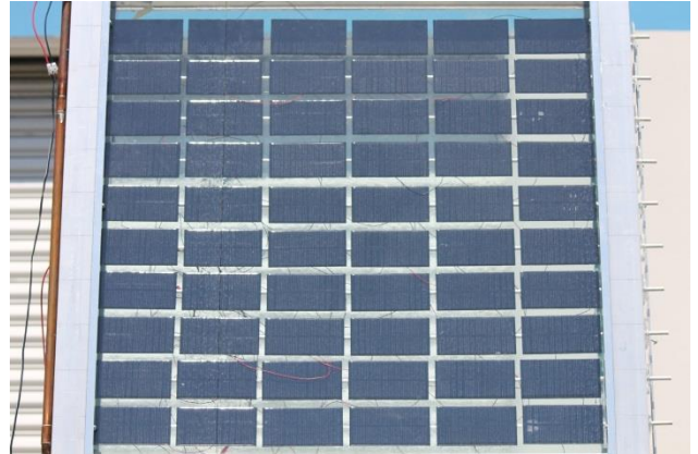
Figure 7: Solar Array located in Prototype III.
